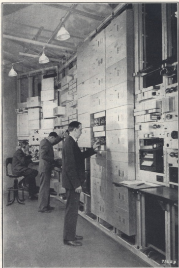
Telephone engineers at the 240 circuit terminal of the experimental coaxial cable system.
