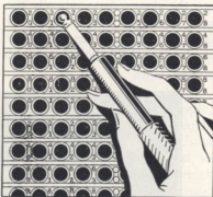
Each of these "jacks" on the switchboard is a door to a subscriber's telephone.
